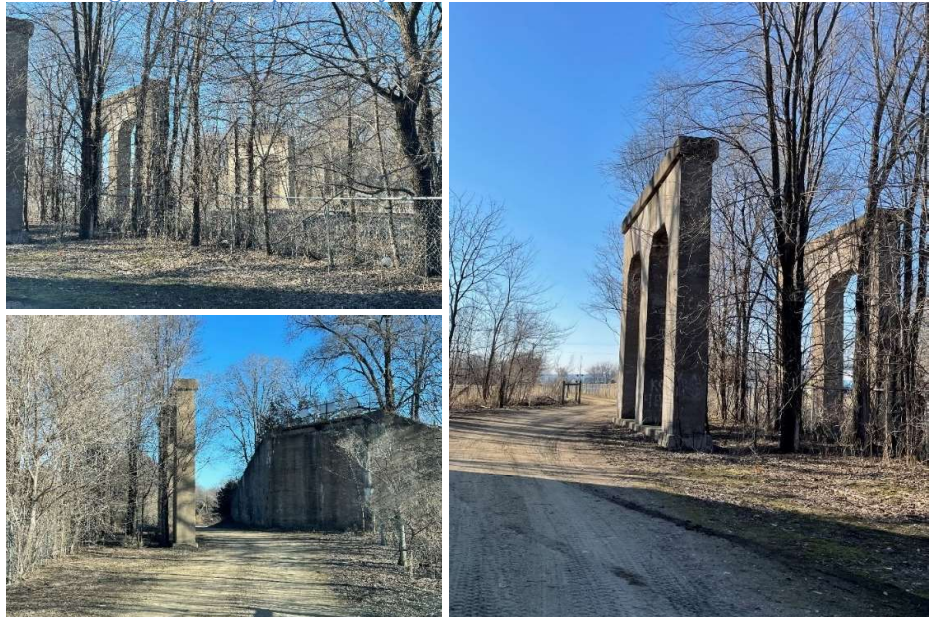
Existing bridge piers previously carried a local road over the CP rail corridor.
